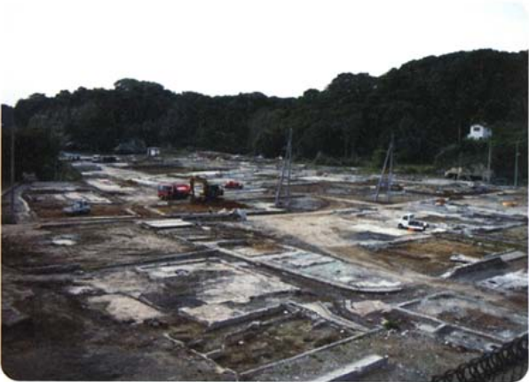
A look at the Tsukihama coast line after the removal of the debris
