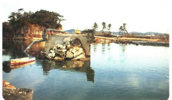
Matsugashima Bridge, the only bridge onto Miyato Island, severed by the tsunami, leaving the island isolated
